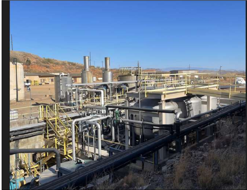
Figure 17-12: JCM Tank Farm
