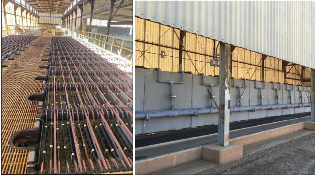
Figure 17-11: JCM EW Tankhouse Interior and Exterior
