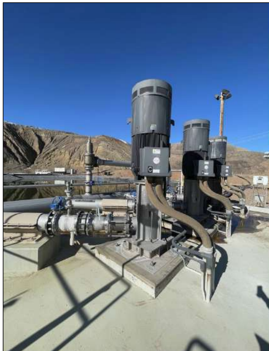
Figure 17-7: Raffinate Pumps at JCM
